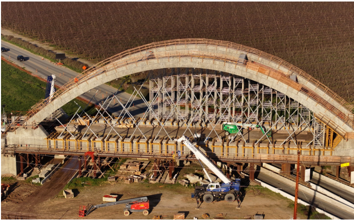
The Tied Arch Bridge in Fresno County will span 249 feet long and will take high-speed trains over State Route 43.
