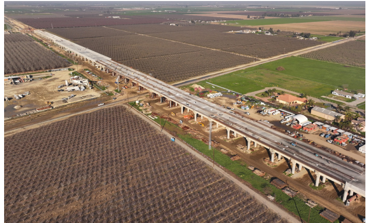
The Hanford Viaduct is the largest project in the 119 miles of construction. It spans more than 6,330 feet and will be home to the future Kings/Tulare Station.
